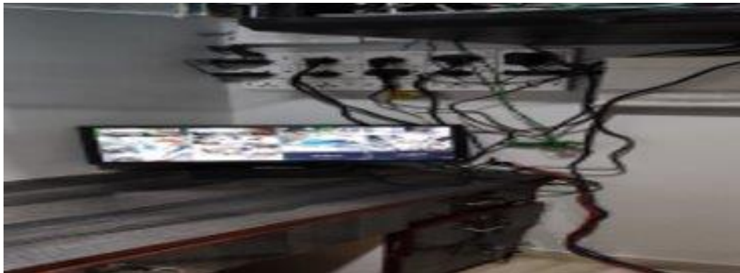
DVR and CCTV Monitor Screen
