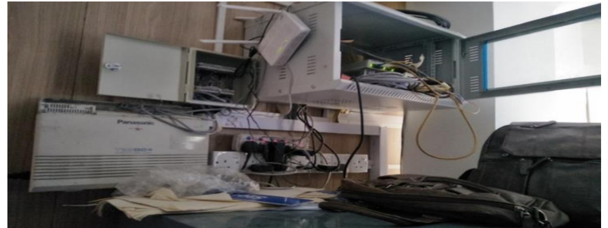
Unmanaged Network Room
