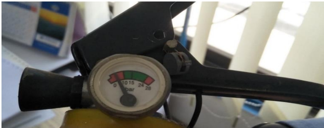
Fire extinguisher - Status
