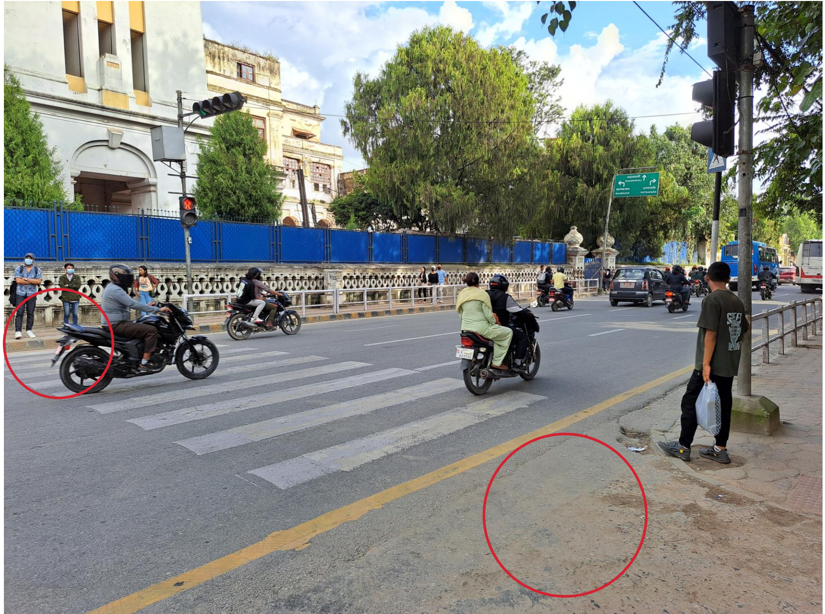
Drop kerb for vehicles but not for pedestrian
