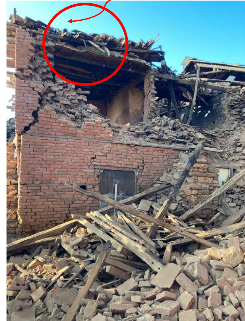
Corner separation, collapse of roof and failure of supporting walls
