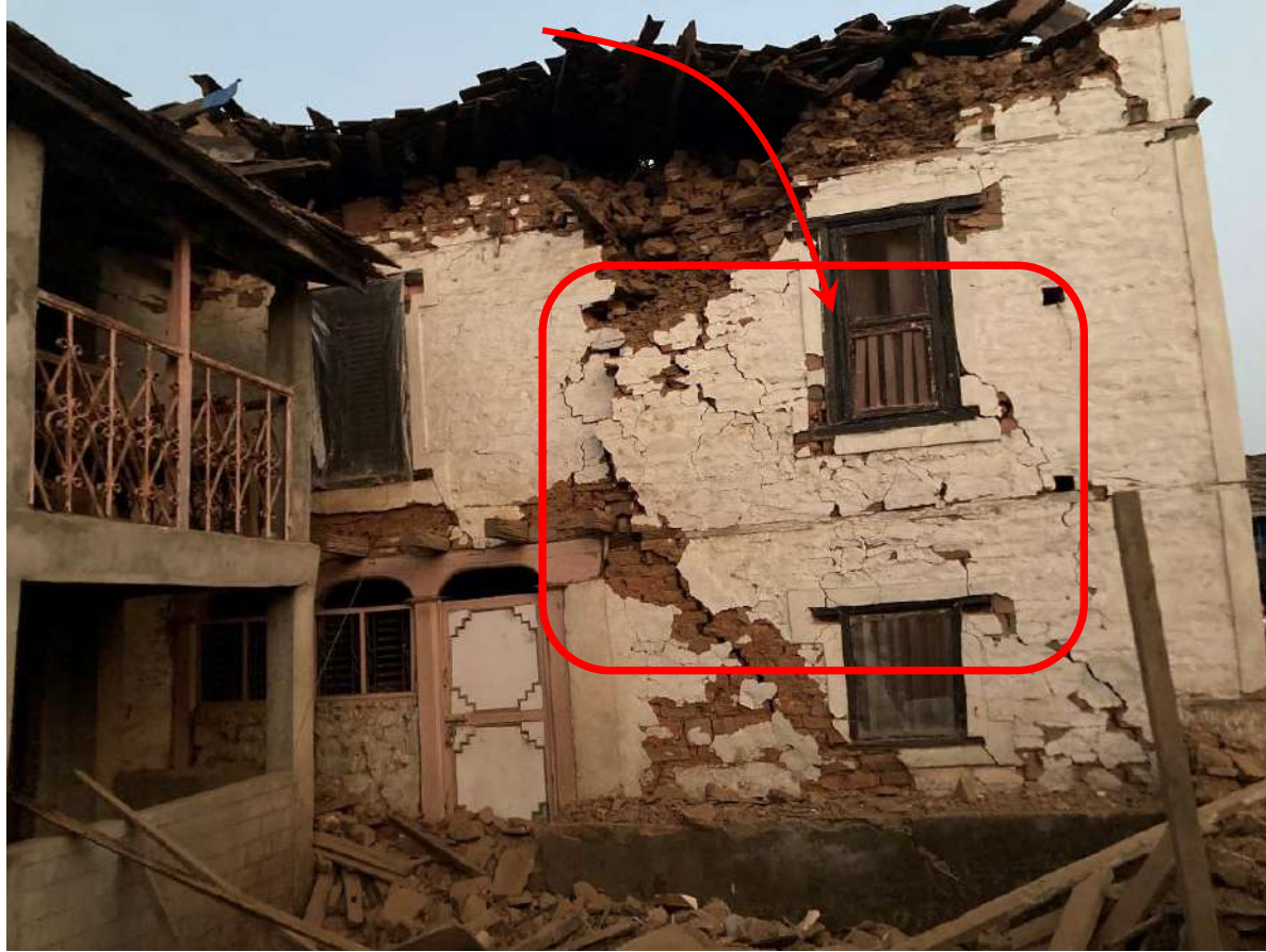
Diagonal shear cracks
