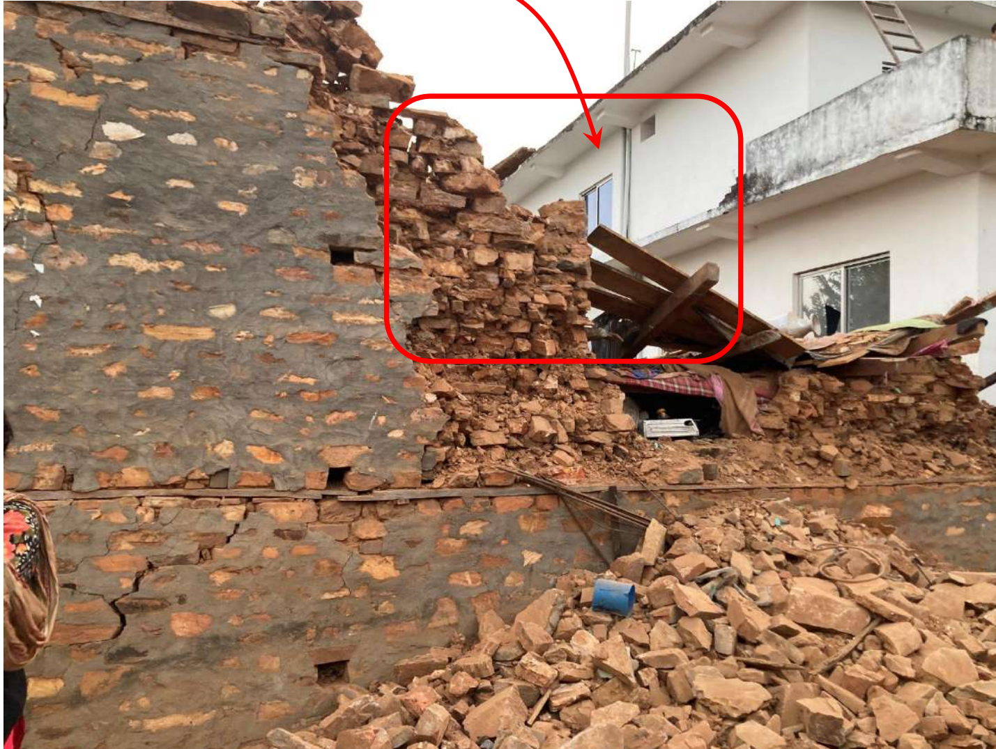
Lack of bonding stones
