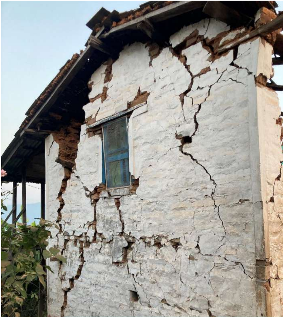
Absence of gable band and heavy roof lead to the formation of cracks at the corners and diagonal cracks in the URM walls leading to collapse
