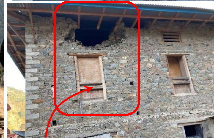
Out-of-plane failure of SMM wall- absence of roof band
