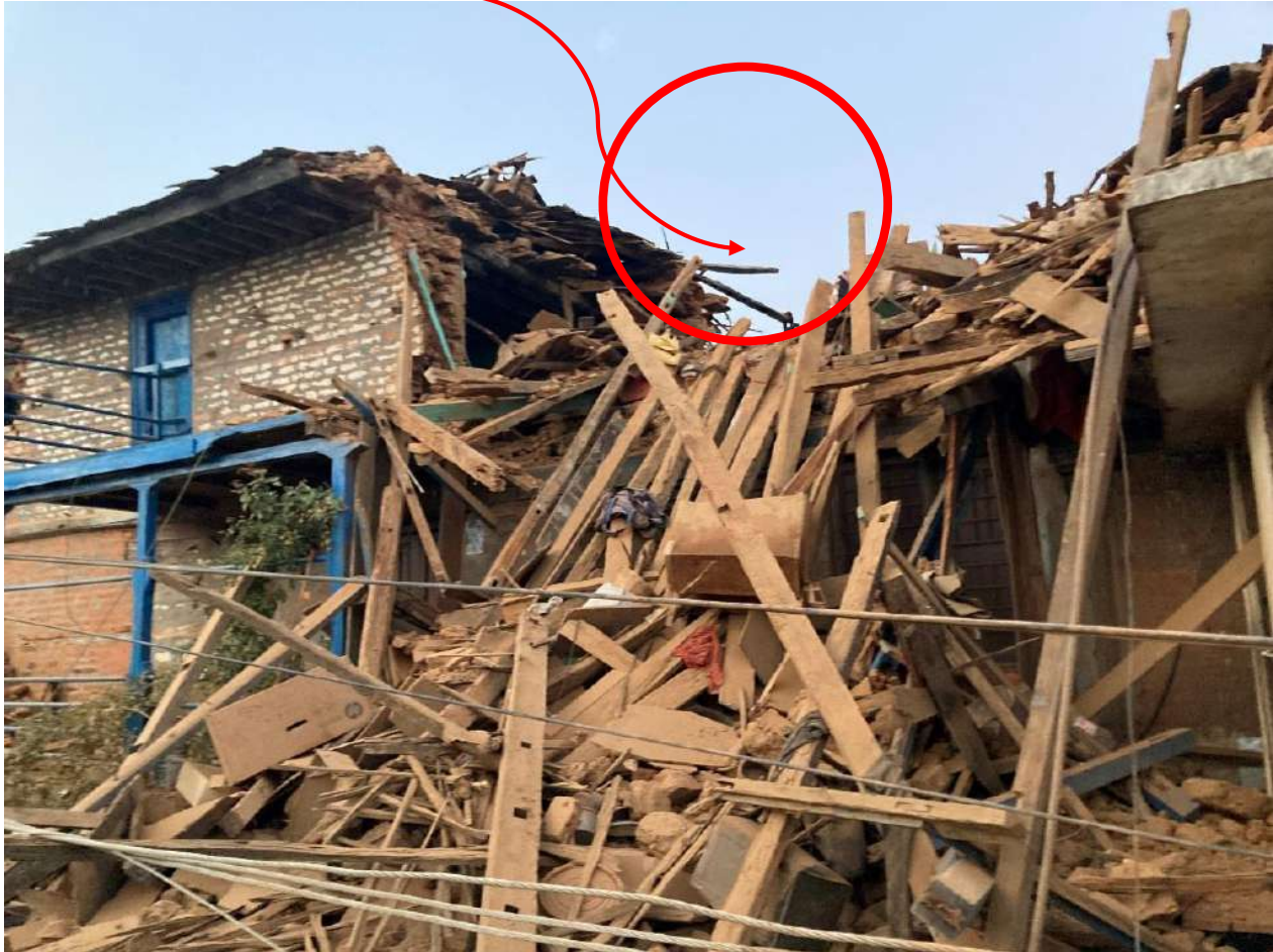
Collapse of roof and failure of supporting walls
