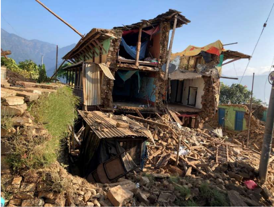
Failure of supporting wall
