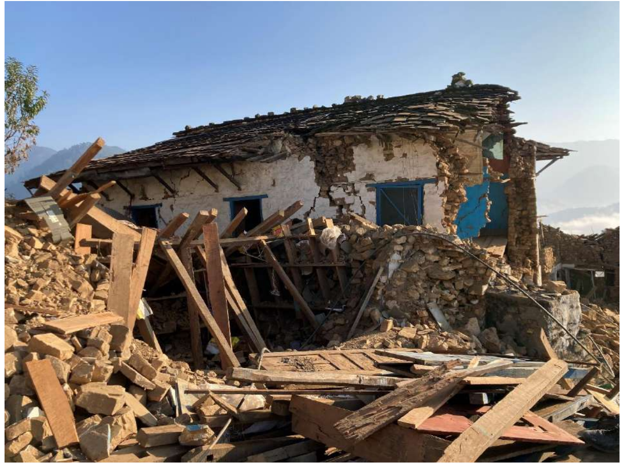
Weak diaphragms and their poor connection with the masonry wall caused collapse of floor as well as failure of supporting walls
