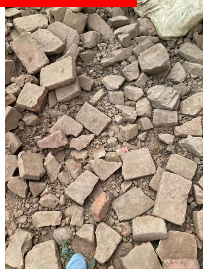
Out-of-plane failure of gable and supporting walls
